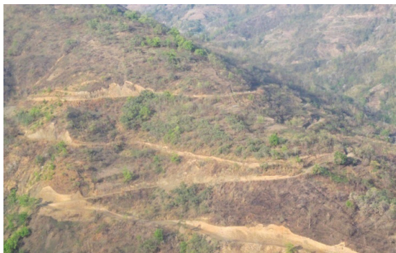
Plate 3: Construction of Agri-Link Road in Murhepu Catchment. Road Construction on the steep hill slopes accelerates soil erosion and landslide below Phusachodu.
